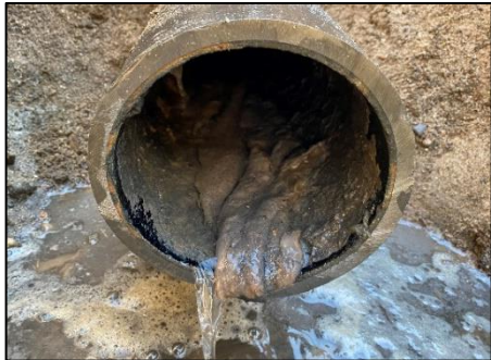
Photo: Distribution System Interior
